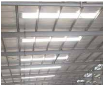
Translucent Panel (Skylight) ↑
