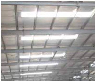
Translucent Panel (Skylight) ↑
